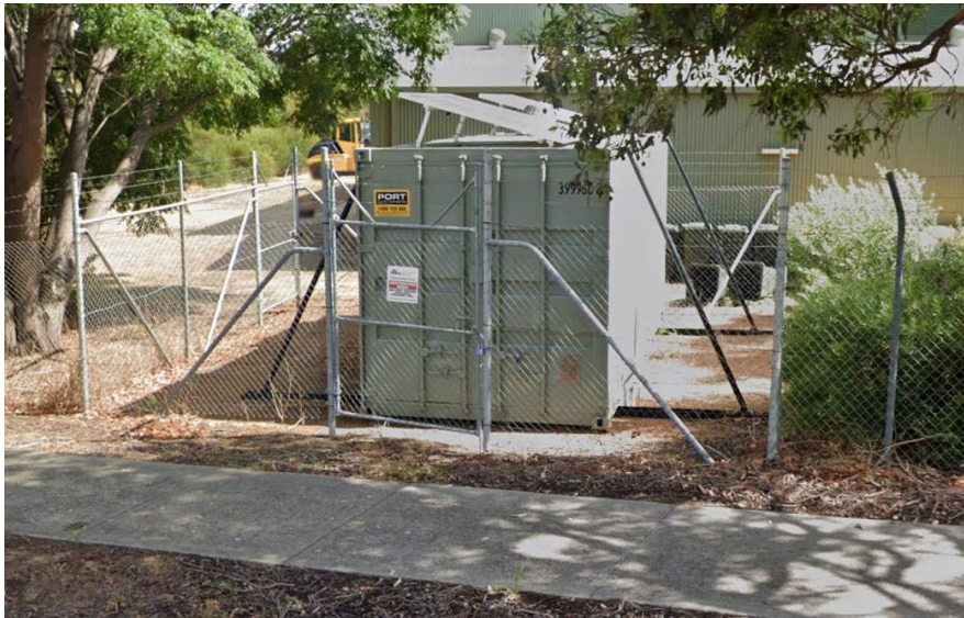
Image 1. Storage container housing the wireless internet repeater equipment. Access from Elliott Street.
