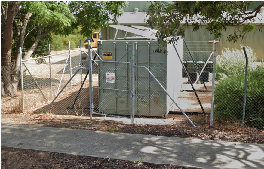
Image 1. Storage container housing the wireless internet repeater equipment. Access from Elliott Street.
