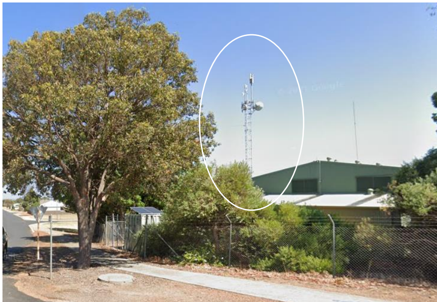
Image 2. Crisp Wireless Pty Ltd antenna infrastructure installed on south-western corner of Depot workshop, 64 Thatcher Street, Waroona.
