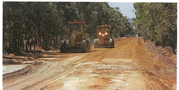
Charlie Eatts and Waroona Earthworks grading the sub base of Coronation Road.
